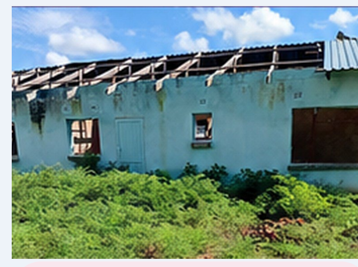
MT DARWIN · STORM DAMAGE
